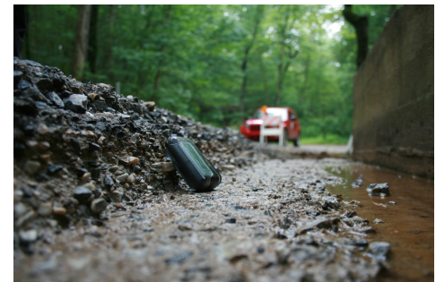
Right: Road damage on a Bentz Rd. bridge. A pager reveals the depth of the erosion.
