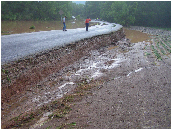
Left: Junction Rd. in North Codorus Twp. outside of Seven Valleys Borough. The water up to the road on the left. The road drops off just as much as on the right side of the picture. Notice the major erosion from the right side of the road.
